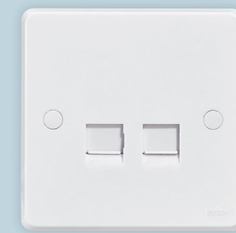
BT master telephone + RJ45 data socket
